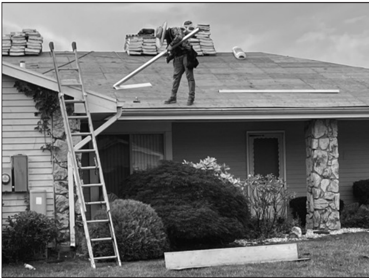
The last house in Section 14 gets a new roof replacement after an eight-year project.
